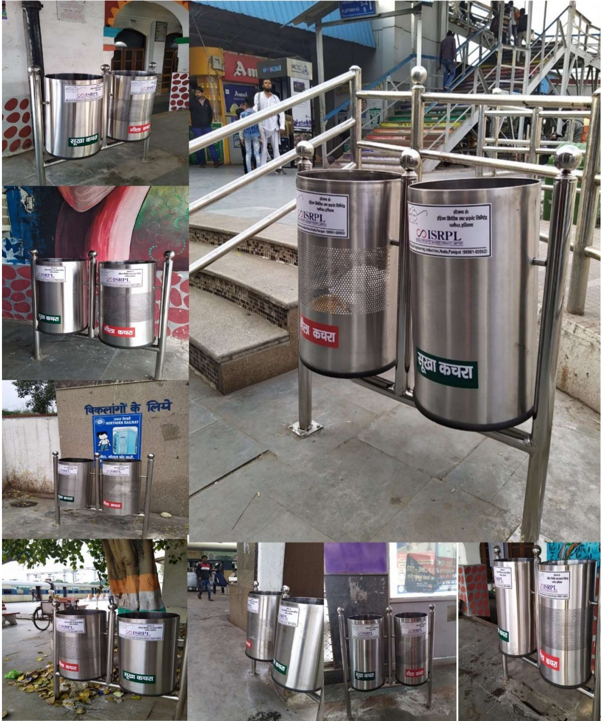
To eliminate open defecation and improve solid waste 10 Nos Segregated Dustbins installed at Panipat Railway Station Panipat (Haryana) under Swachh Bharat Mission of Govt. of India as CSR initiative by ISRPL in FY 2019-20
